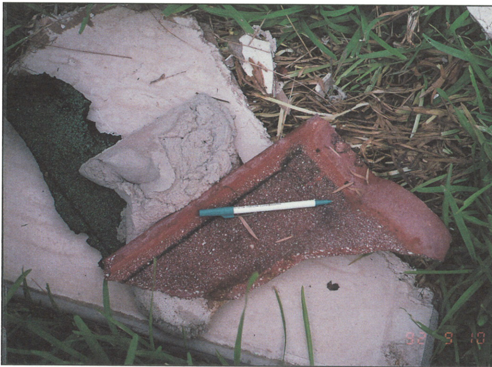
FIGURE 22. Typical failure of roof sheathing-to-underlayment attachment. (Bond between underlayment and mortar pad, and between mortar pad and tile effective.)
