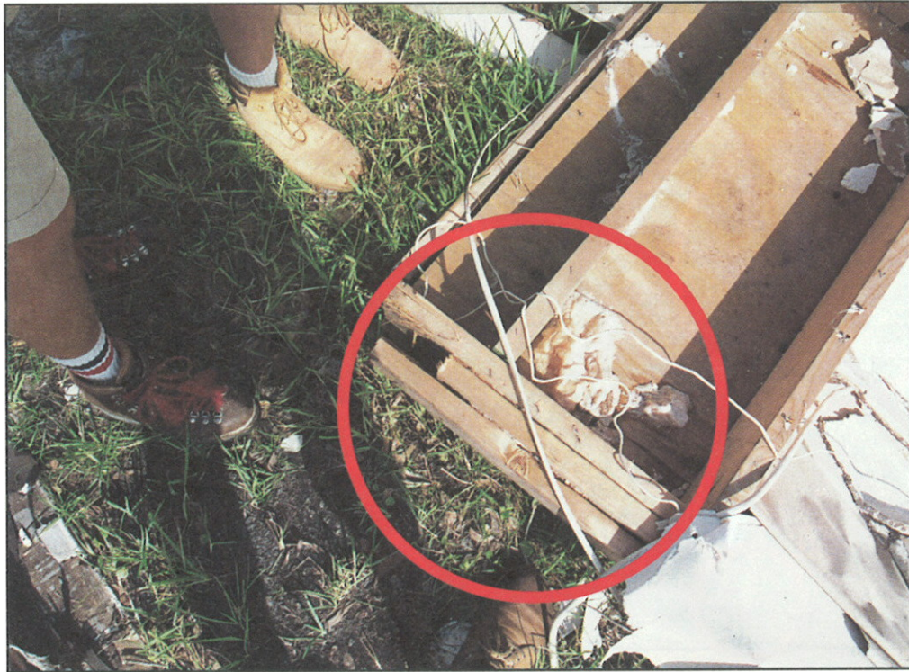
FIGURE 10. Top plate splice not able to transfer horizontal loads.
