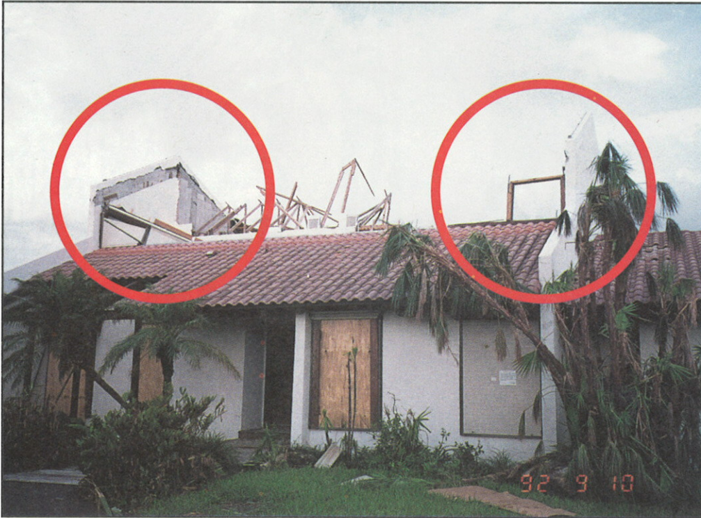
FIGURE 17. Two-story masonry building. While forces were sufficient to blow off entire roof structure, continuous masonry gables held.
