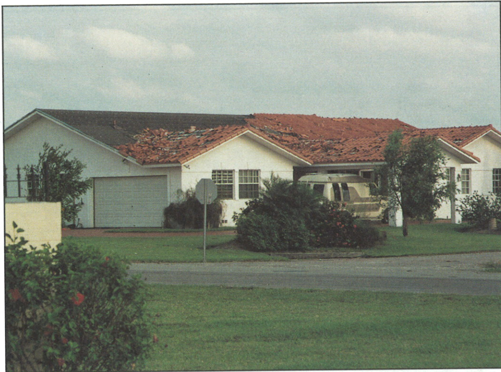
FIGURE 36. Failure of barrel tile roofing. Bond failure between underlayment and mortar and between mortar and tile was observed.
