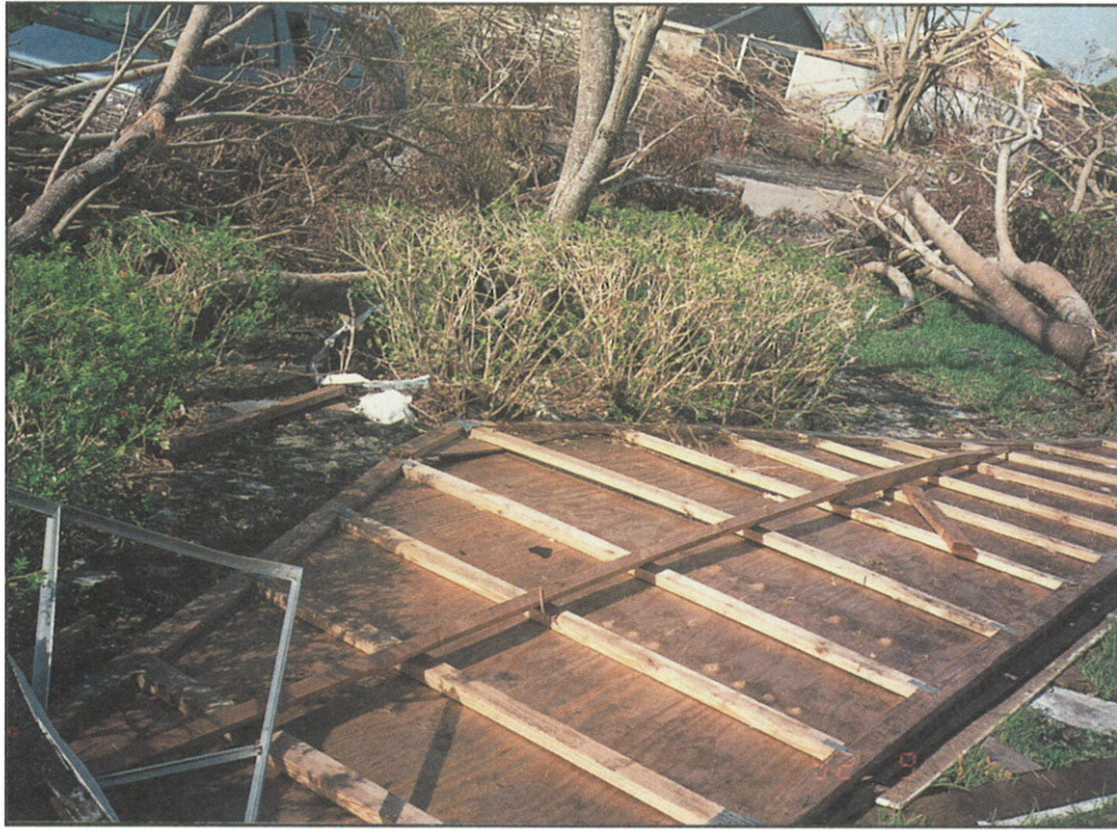
FIGURE 6. Entire wood gable separation. Bracing connection, if completed, may have prevented this from occurring.
