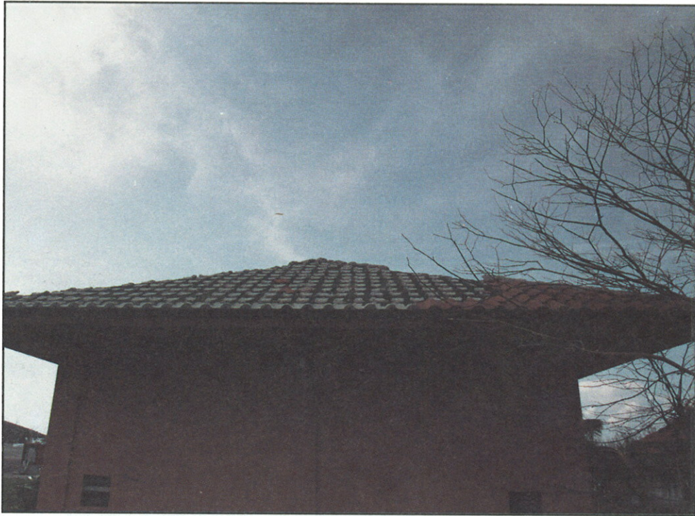
FIGURE 34. Failure of "S" tile roofing. Bond failure between mortar and tile was observed.
