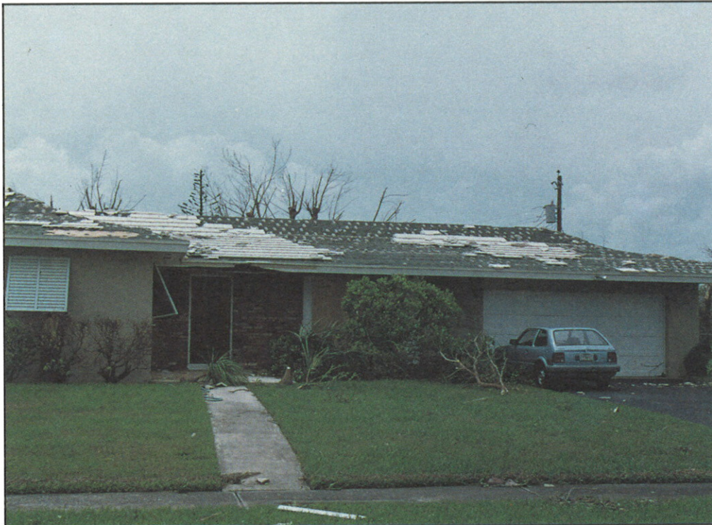
FIGURE 32. Failure of extruded concrete flat tile roofing. Bond failure between tile and mortar and between mortar and underlayment was observed.
