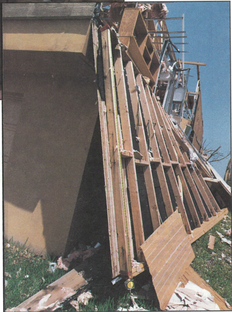
FIGURE 60. Side wall failure. Side wall has no lateral load transfer capacity due to inadequately built-up corner post.
