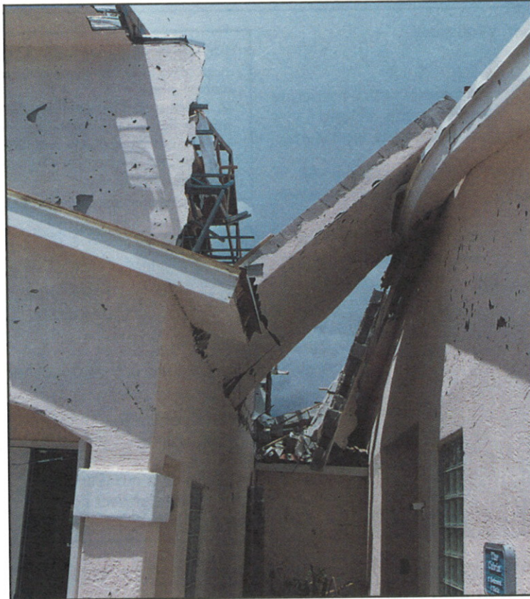
FIGURE 67. Firewall separation . Results from building corners being discontinuous with tie- beams. (See Figure 68 for side view)
