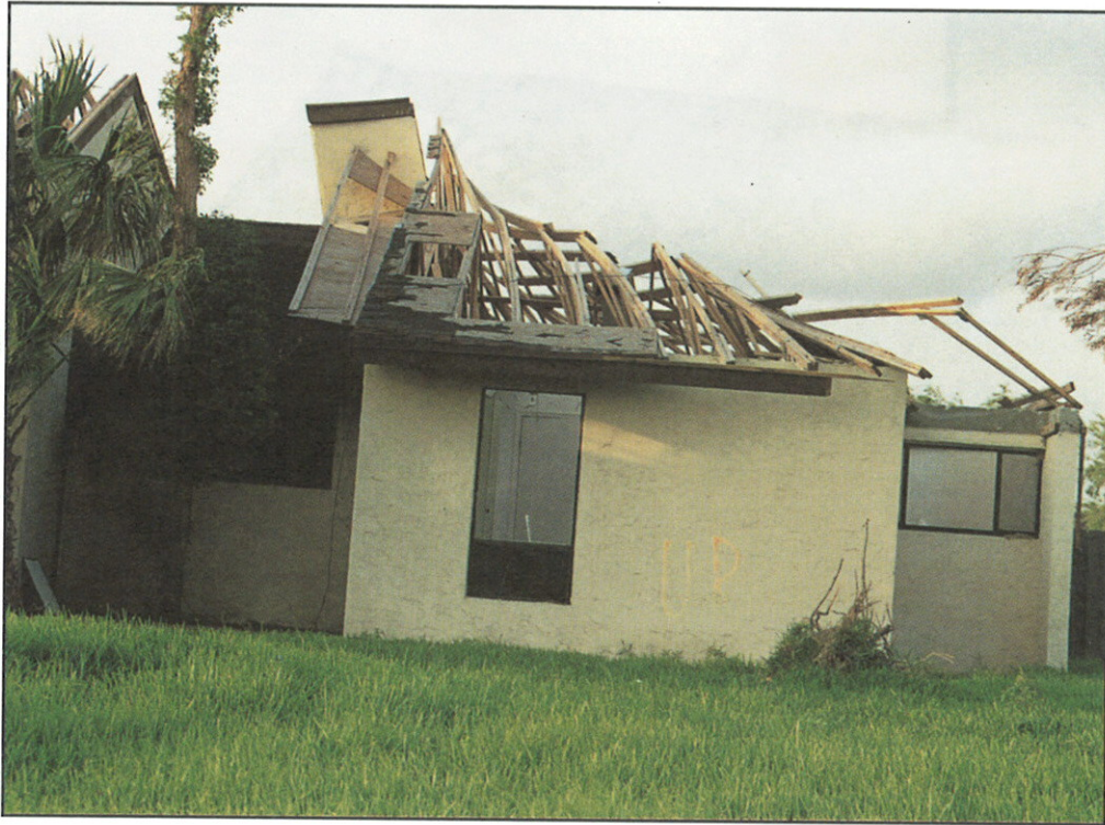
FIGURE 14. Roof structure failure due to inadequate bracing.
