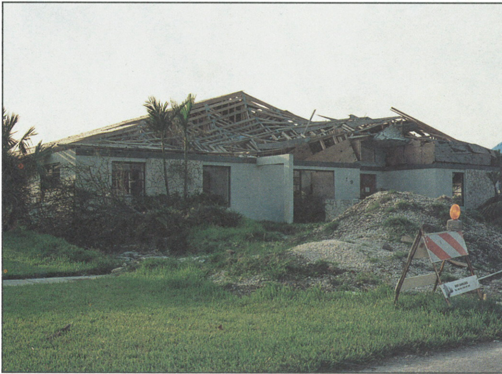
FIGURE 7. Typical gable failure. Inadequate bracing support and ridge blocking evident in inward collapse.
