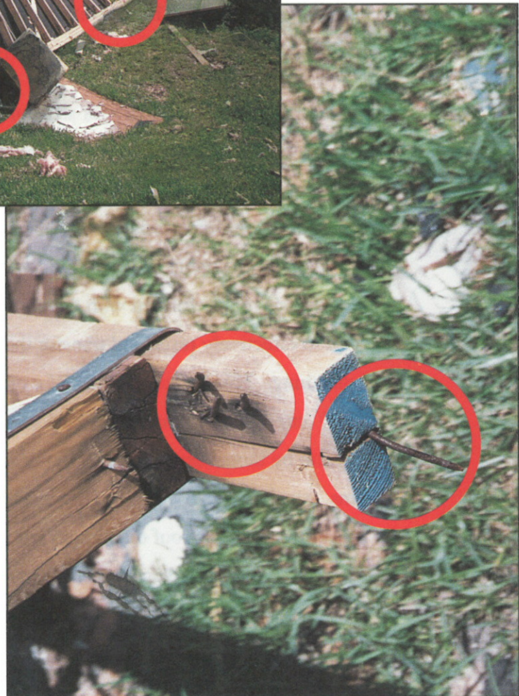
FIGURE 5. End of exterior non-loadbearing wall top plate. Transfer of forces on entire wall depended on a limited number of nails.
