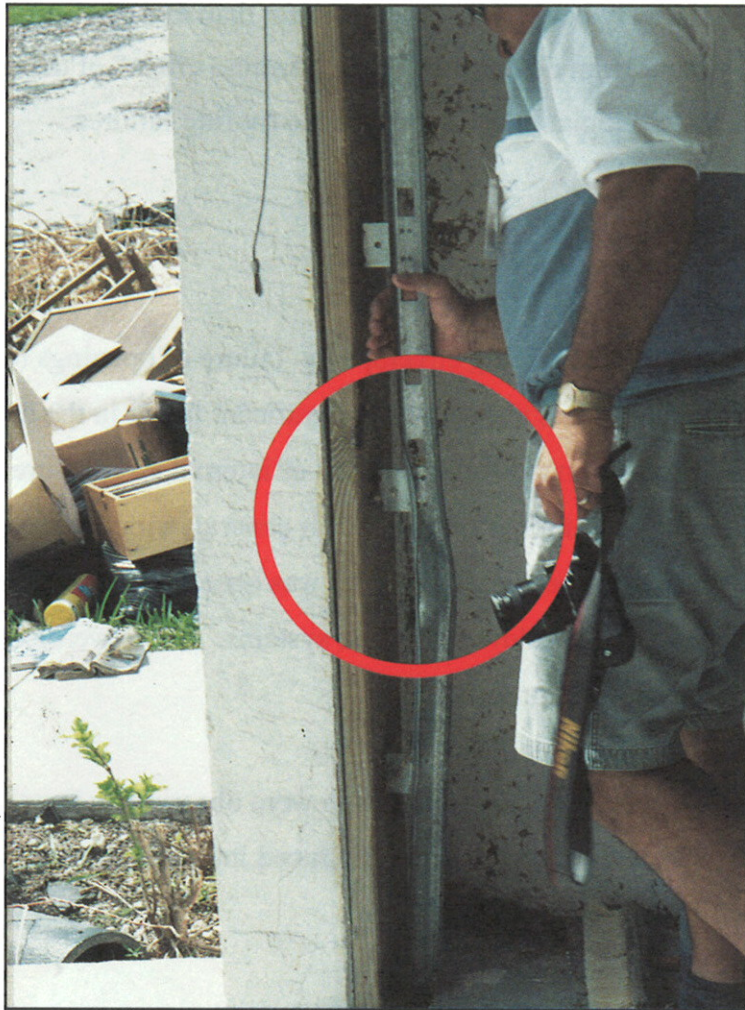
FIGURE 25. Garage door failure. Rotation of track, and pullout of brackets at wall support.
