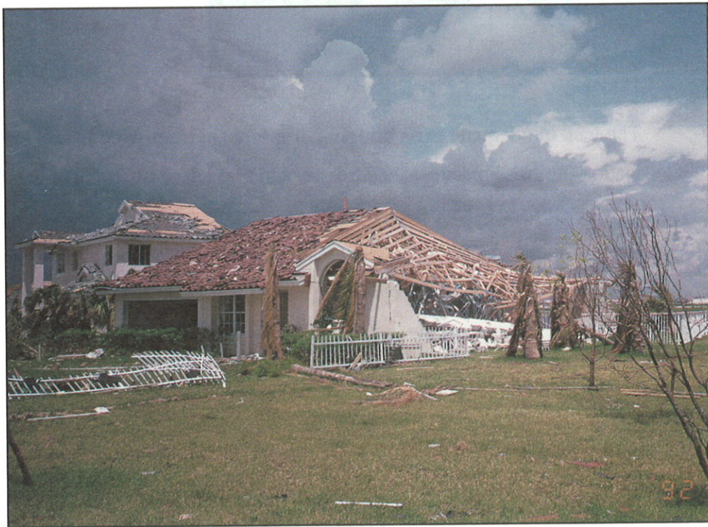
FIGURE 13. Roof structure failure due to inadequate bracing.
