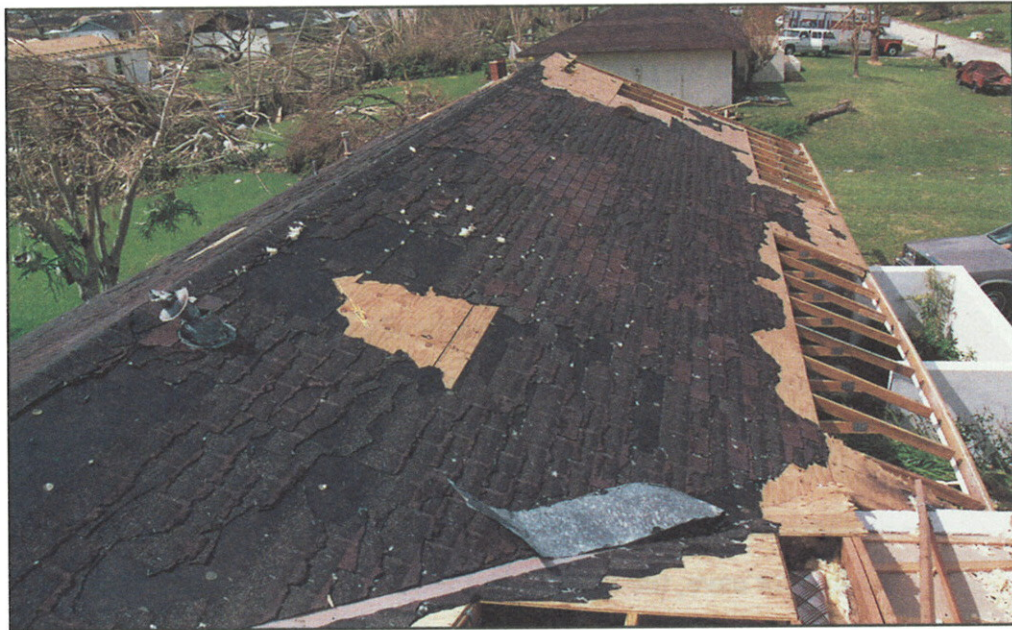
FIGURE 30. Composition shingle and underlayment failure.
