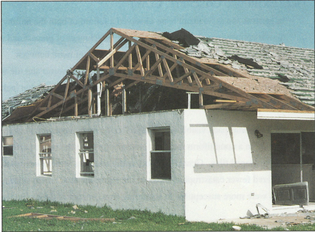
FIGURE 23. Typical roofing failure. Failure of sheathing, underlayment, and extruded concrete tiles.
