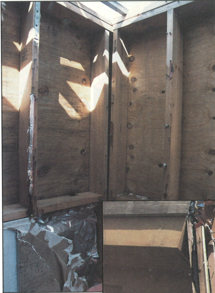
FIGURE 59. End column/corner post missing from wall.
