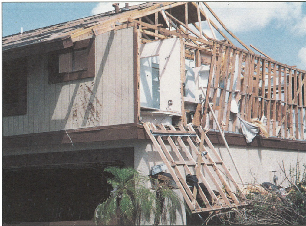
FIGURE 18. Second story wood framing (on first story masonry). End gable and wall failure.
