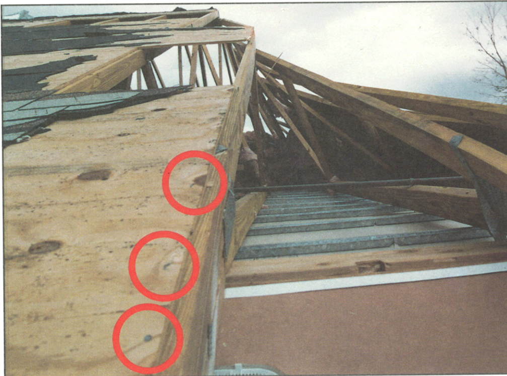
FIGURE 57. Sheathing only tack-nailed.
