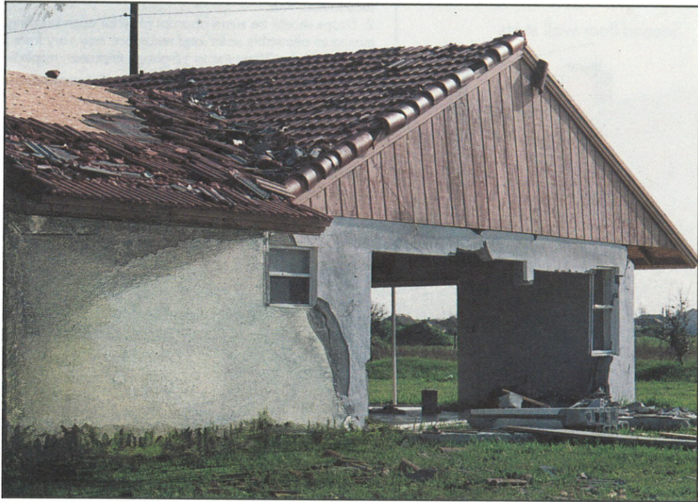
FIGURE 63. Example of masonry construction. Wall separated from building envelope due to inadequate vertical wall reinforcing in connection to horizontal tie-beam.
